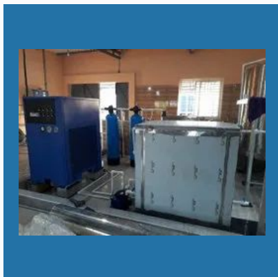
Water Online Chillers
